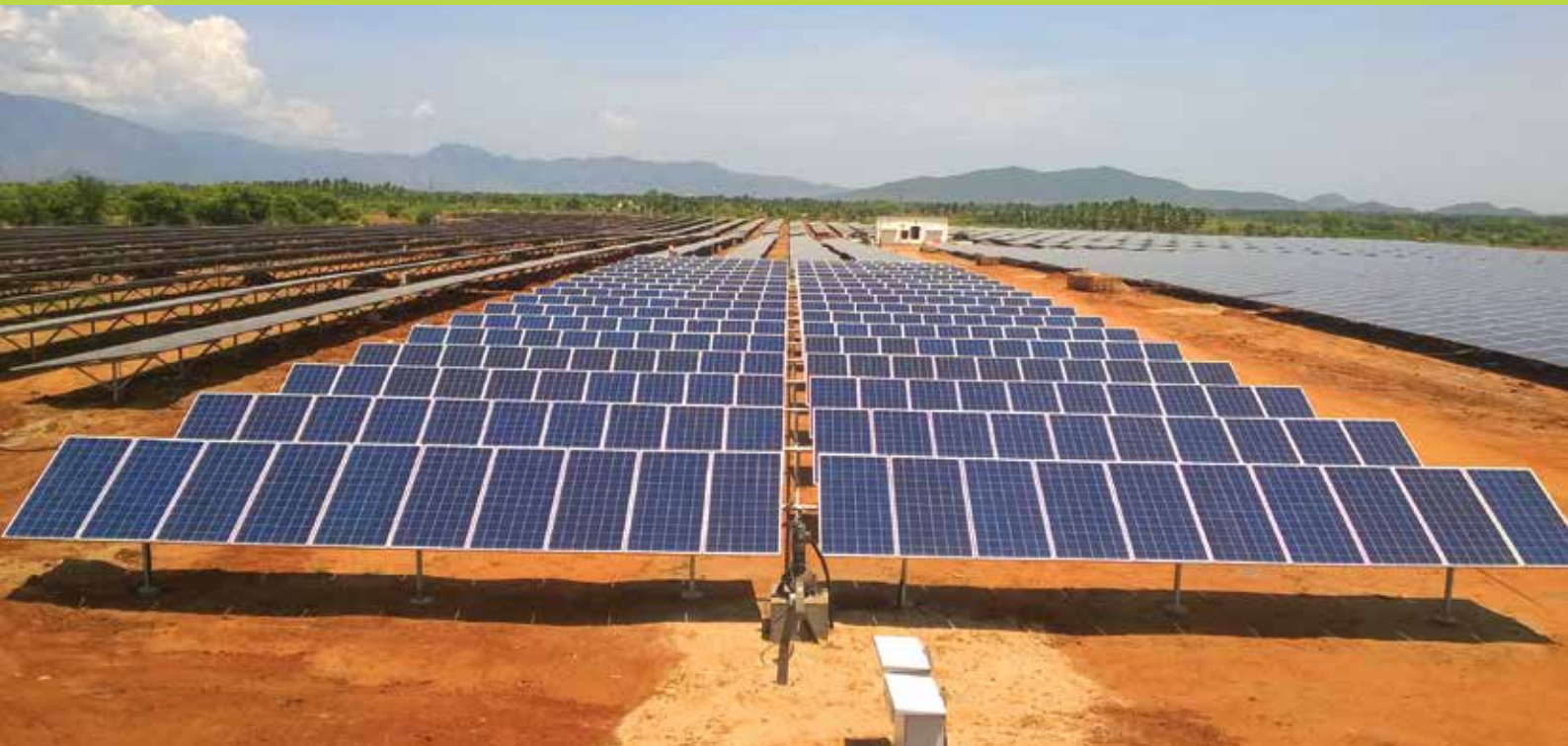
India's single largest solar tracker plant with a capacity of 60MWp in Tamil Nadu, 2016, constructed by L&T.
